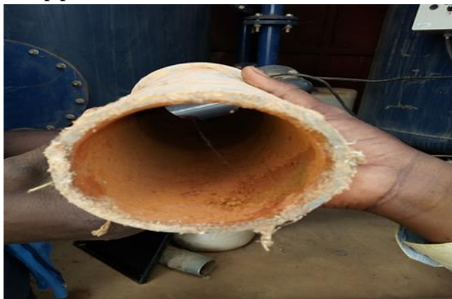
Figure 1: Photo of iron tartar in the Dan Daji -Illéla water distribution pipes.
